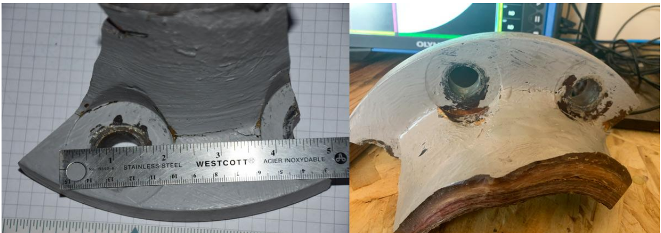
Figure 2. Cracking between bolt holes in a sample cut from an FRP flange
